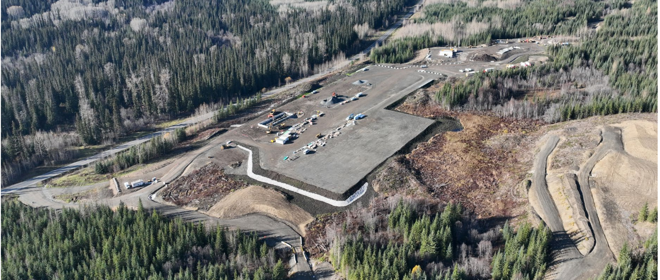
BC Hydro's Treaty Creek Terminal
