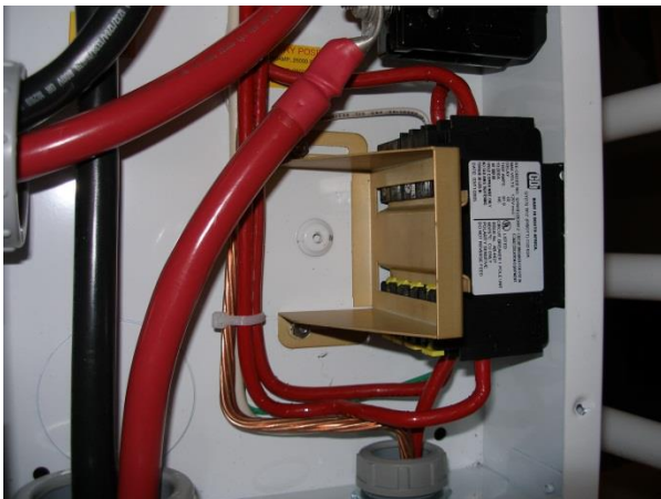
Din Rail mounted breakers
