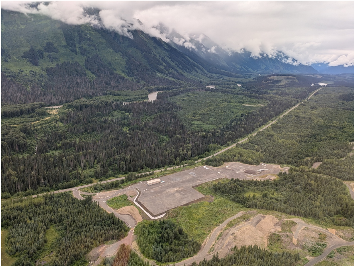
Substation site at Seabridge Gold's KSM in British Columbia, Canada (Photo: Paul Harris)
