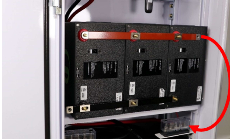
Figure 8.0 - PHI Battery Wiring Using Interconnecting Busbars
