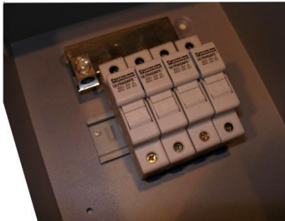
4 Touch safe fuseholders installed in an MNPV6
