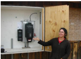
A Positive Energy installation, NM Outdoors in an enclosure
